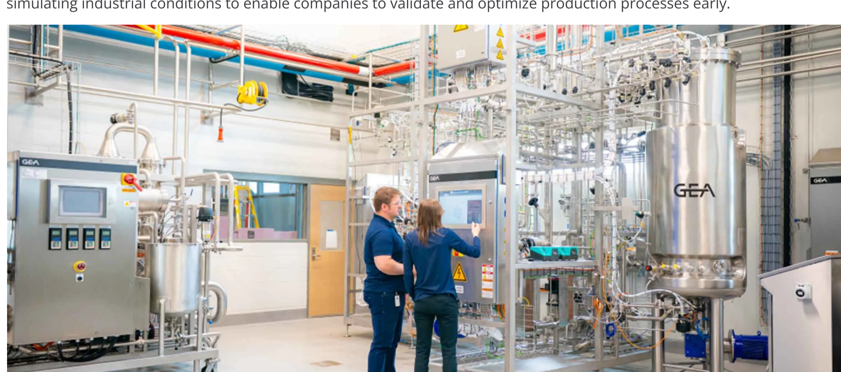
GEA recently opened an innovation center for precision fermentation and cell cultivation in Janesville, Wisconsin. Image courtesy of GEA.
