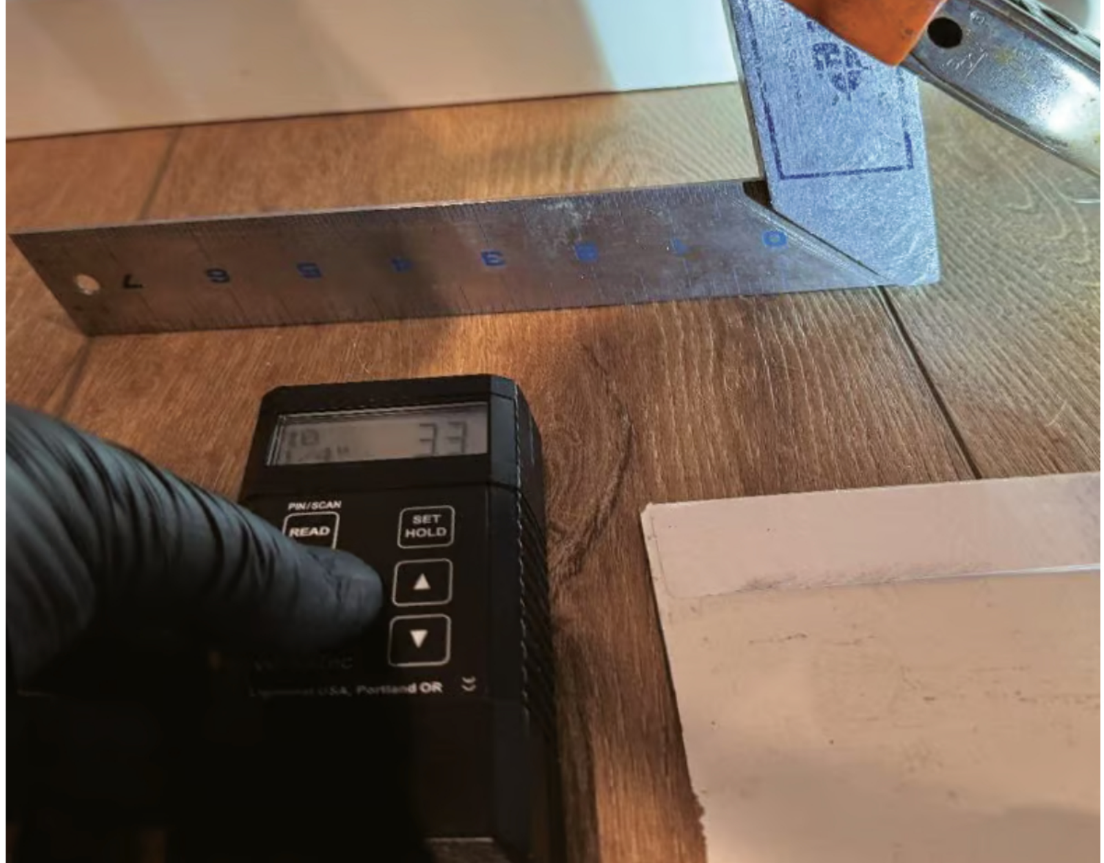
In comparison, areas showing values around 3.3 had no visible defects. The correlation was clear: the higher the moisture reading, the more severe the damage. Photo: Lignomat.
