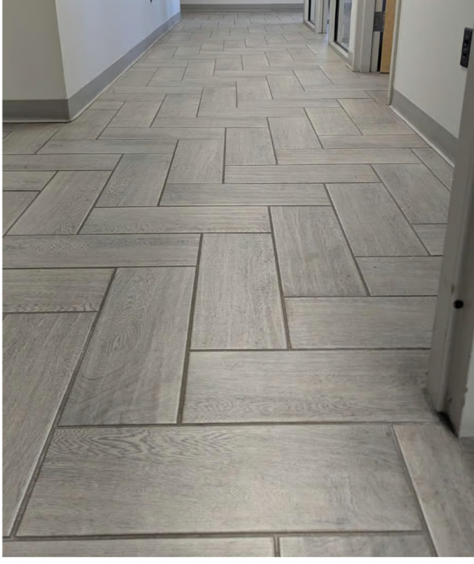
At first glance, this herringbone pattern seems acceptable. However, closer inspection reveals misaligned long-side grout joints that drift rightward, compromising both the pattern's visual integrity and proper installation standards. Photo: Scott Carothers.
